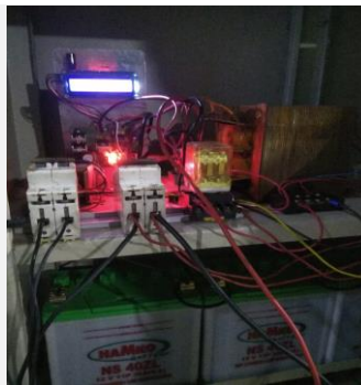
110VDC Battery Charger of Substation
